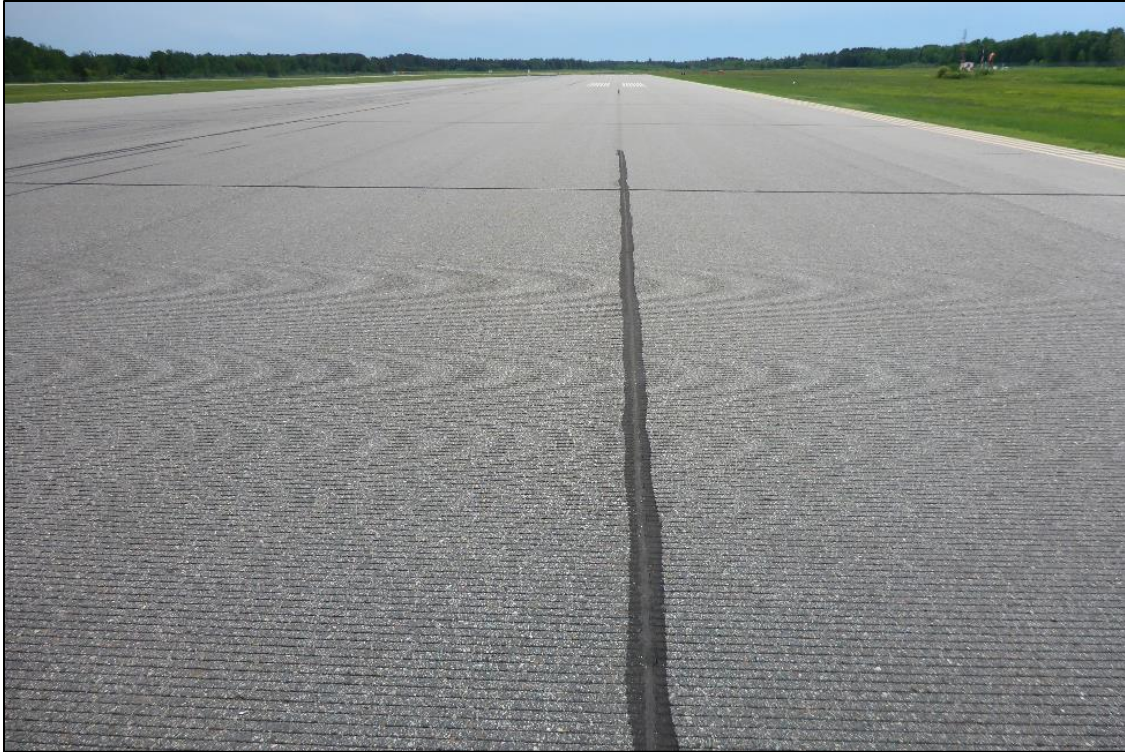
HIB RY1331 004_ (PCI = 88)
